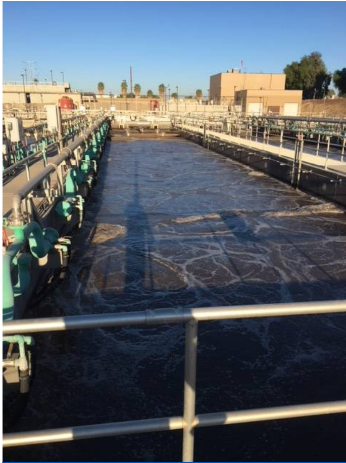
Aeration Basin in Service
